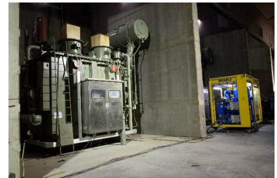
The first 12 transformers are already located at the Transformer Cavern.
