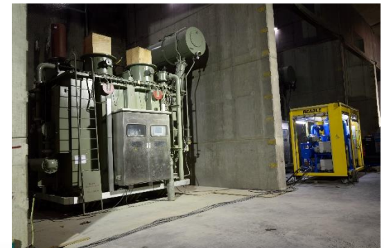
Transformer Cavern: the assembly of the 12 transformers at the North Area is at 99%.
