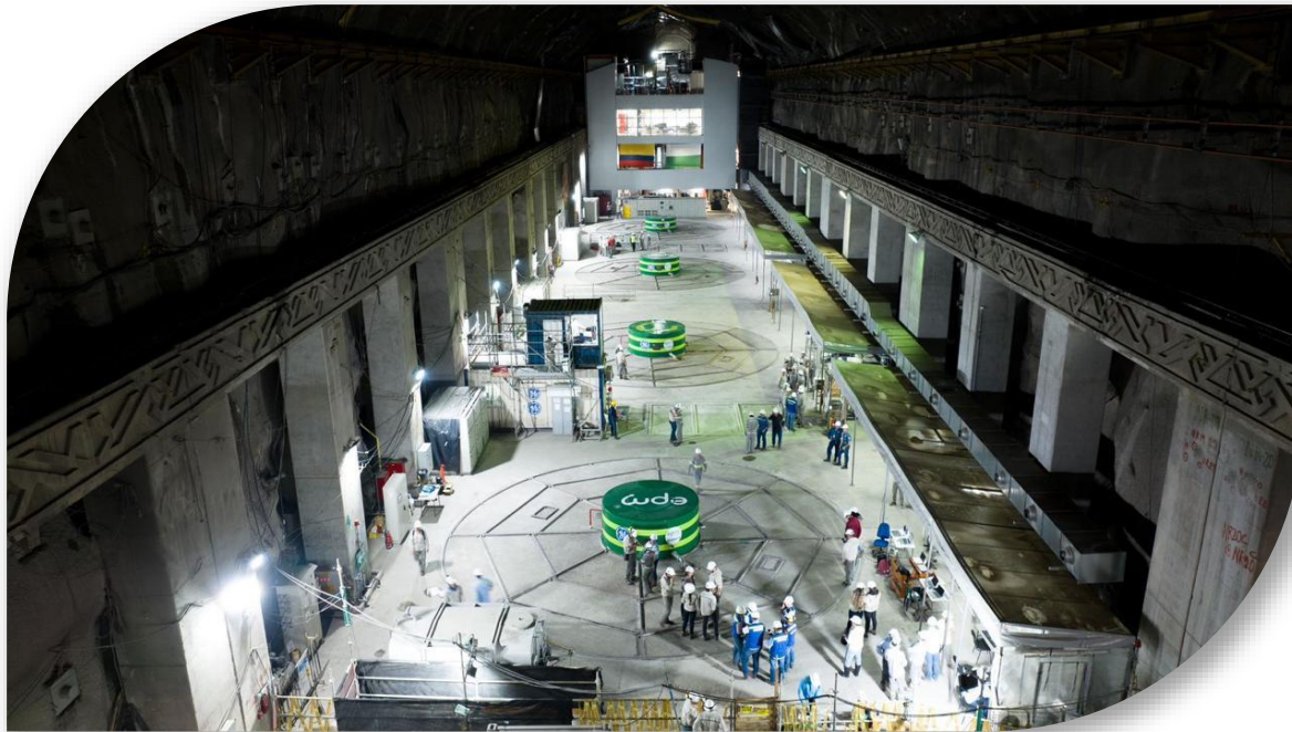
Powerhouse North Zone: Units 1 to 4.
