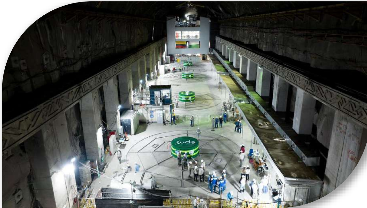
Powerhouse North Zone: Units 1 to 4.
